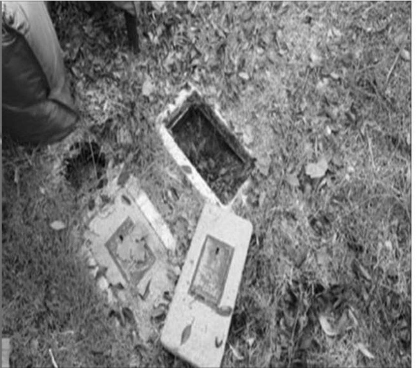
Figure 3: Results of Field Survey Showing Meter Type, Box Condition, and Lid Type
